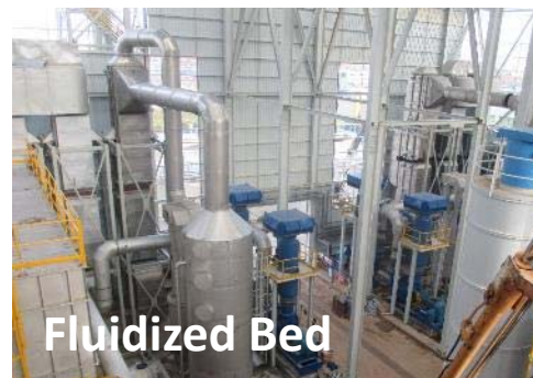
Photo Source: Kuzu Grup, Fluid Bed - http://www.kuzugrup.com/en/proje/buski-fluidized-bed-sludge-incineration-and-energy-production-plant/
